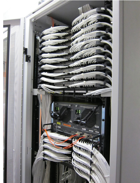
10 G/bs + ready cabling technology powers the Duke-NUS communications network
